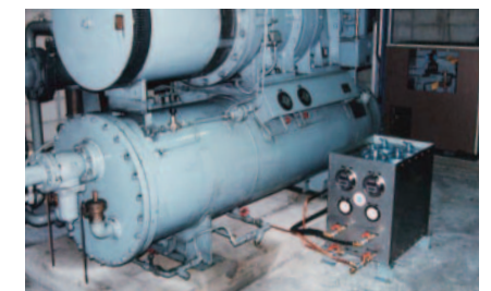
Lubricating oil for the 150 kw screw compressor (SRC-814-C)
